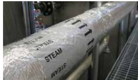
Insulation on steam pipe
