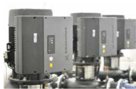
Variable speed drives
