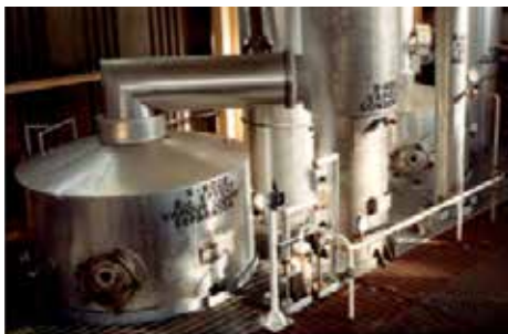
Thermal vapour recompression system
