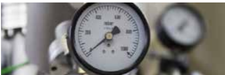
Use the lowest discharge pressure setting possible
